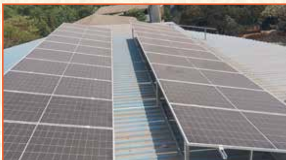
Solar panels installed at Navde High School to support greener infrastructure.
